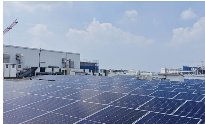
Solar panels installed at the Suzhou Plant
